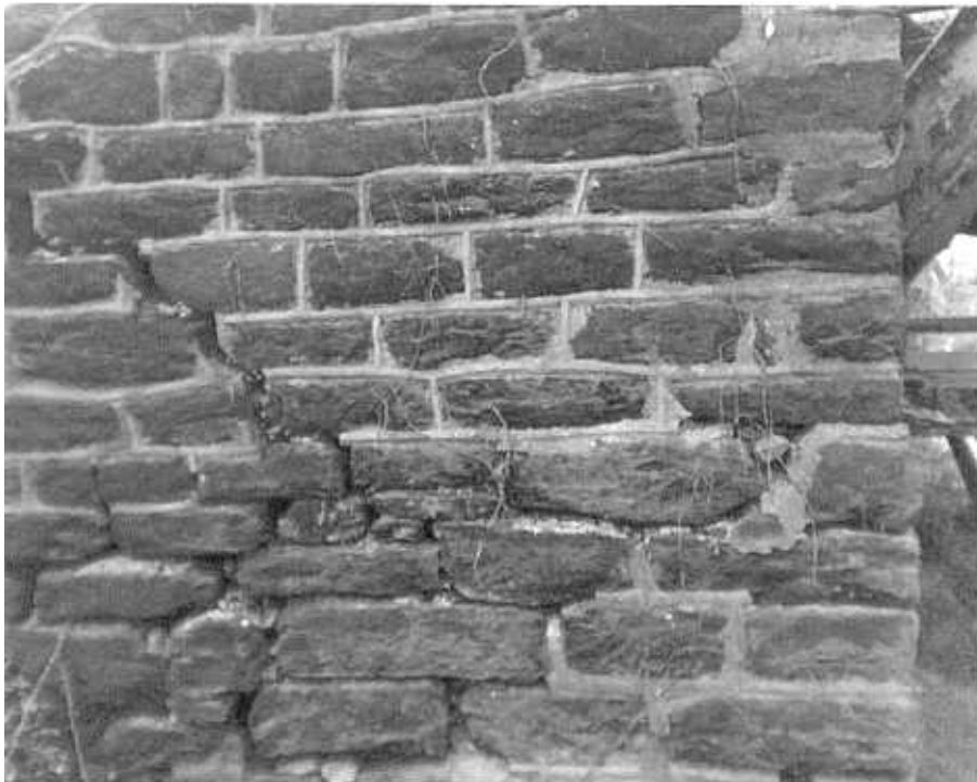
Photo 2 – Loss of mortar on north abutment.
