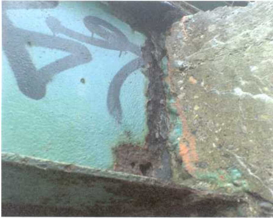
Photo 3 – Deterioration of steel beam encased in concrete at abutment.
