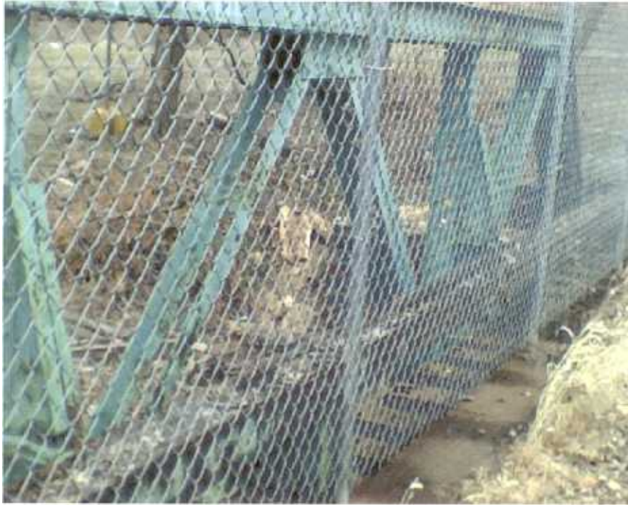
Photo 5 – Looking at chain link fence. This fence does not meet current design requirements.
