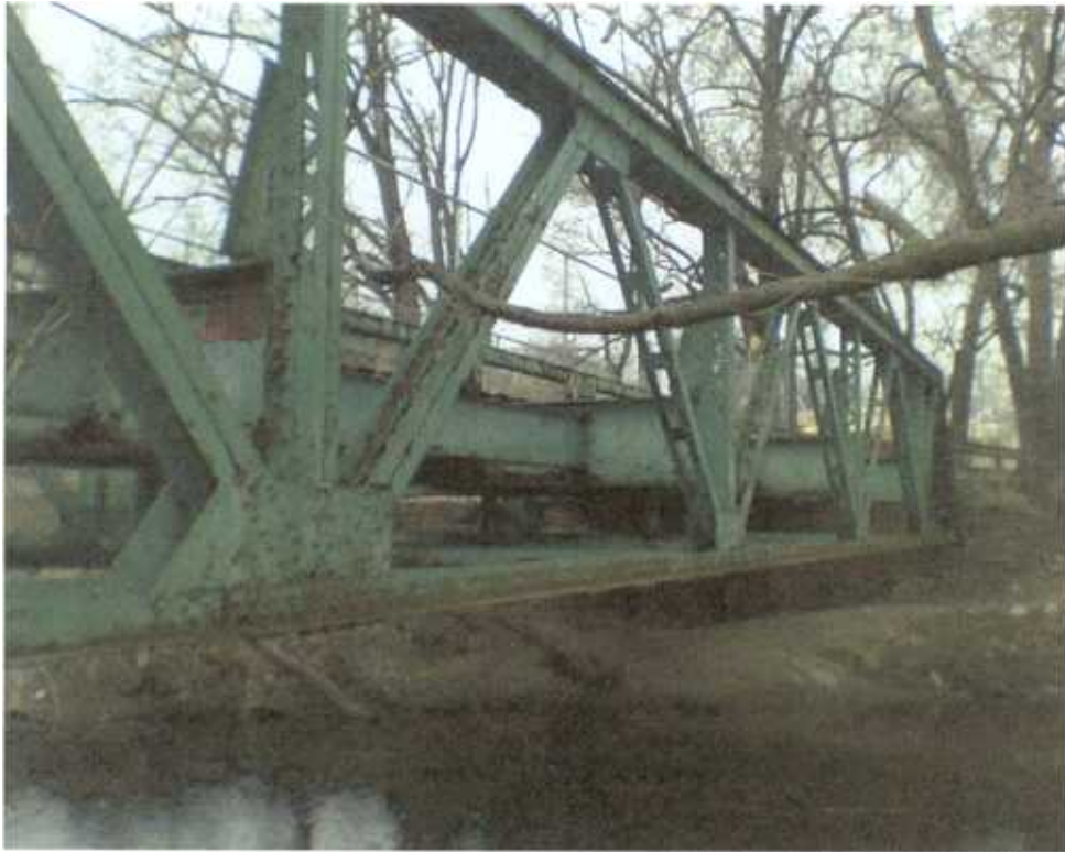
Photo 1 – Elevation of existing bridge. Note peeling paint on truss.
