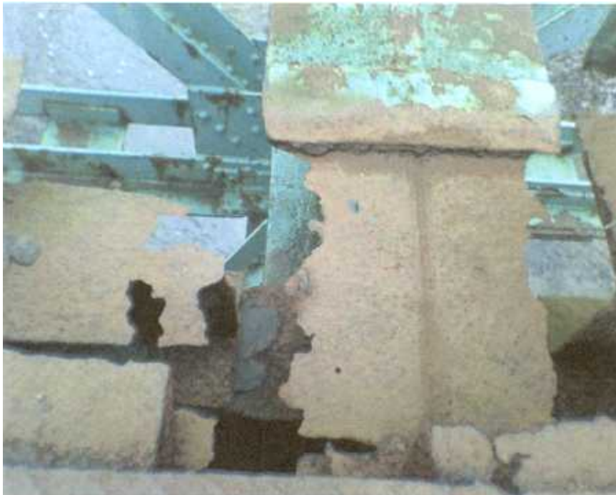
Photo 6 – Looking at top of floor beam at north end of bridge. Note deterioration of top flange.
