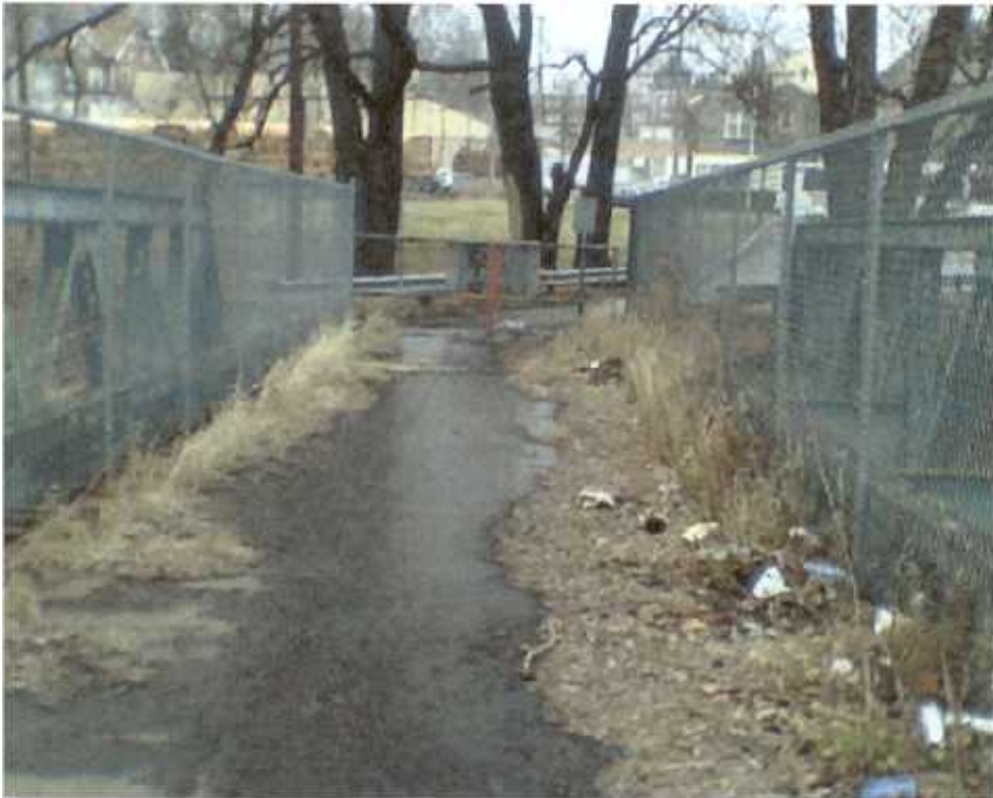
Photo 4 – Looking south at steel deck. Note debris that collects due to flooding and leaves.
